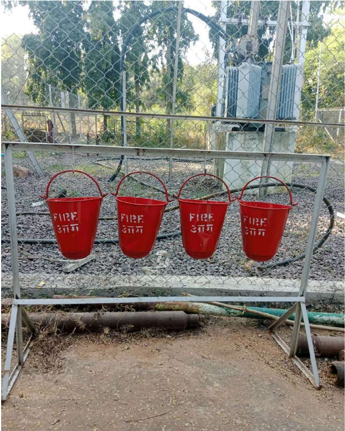
Fire Protection At Site
